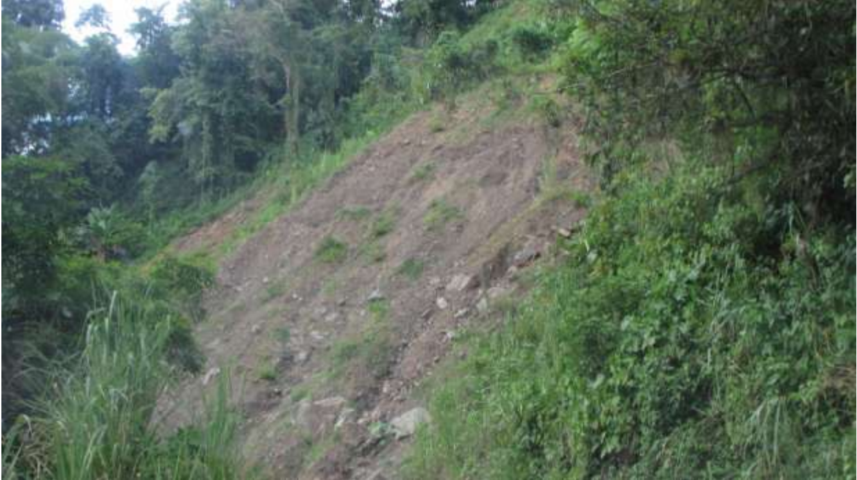
Figure 59: Landslide, Balcarres. Note that the area surrounding it was apparently deforested, which probably contributed to the problem.
